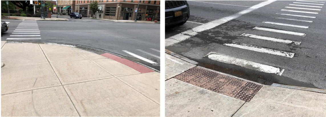
Figure 3.1 – Glen/South/Bay intersection striping and sidewalk ramp condition
