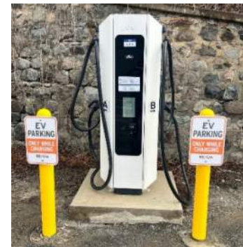
Figure 3-11: DCFC charging station at Warren Ford. Source: www.plugshare.com
